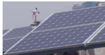
Fig. 16 Installed WEBEL 2300 250W Module
