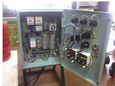
Fig. 8 Control box with all components for operating the 3-phase induction motor on single-phase power
