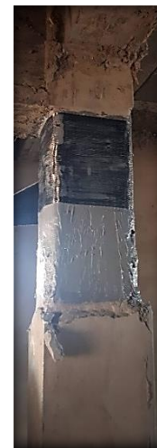
Fig. 1 Reinforcement of critical column areas with CFRP in a building under construction in Beni-Mellal, Morocco
