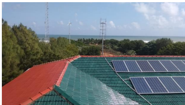
Fig 2: Solar PV module Setup
