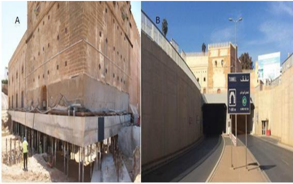
Fig 2. Illustration of the provisional phase (A) and the final state (B) of the tunnel [20, 21].
