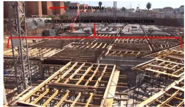
Fig 3. Project site for the construction of the underground parking lot at Bab Lhad Square
