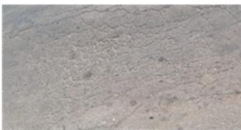
Fig. 1 Fatigue (alligator) cracking
