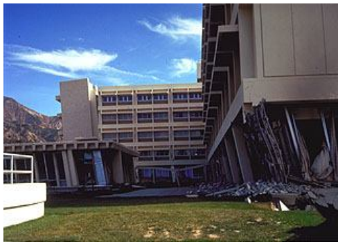
Figure 2 L-Shaped Plan of Commercial Building with Collapse Part
