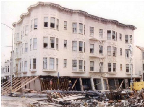
Figure 1 Collapse of Multi-Storey Building Due To Soft Storey
