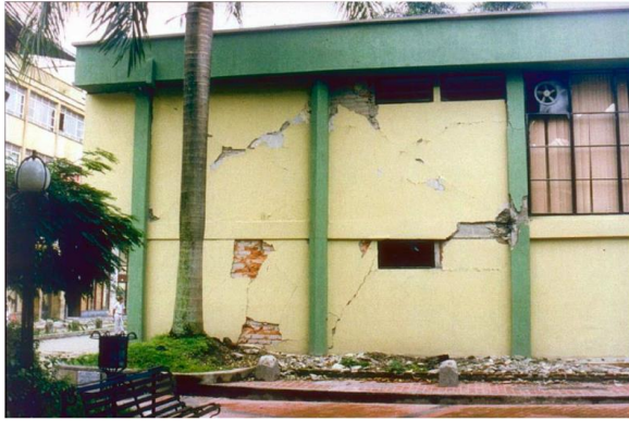
Fig. 1 Major damage to the unreinforced masonry walls and moderate damage to the columns of an R/C municipal building (Quindia, Colombia 1999 Earthquake, EERI) [11]
