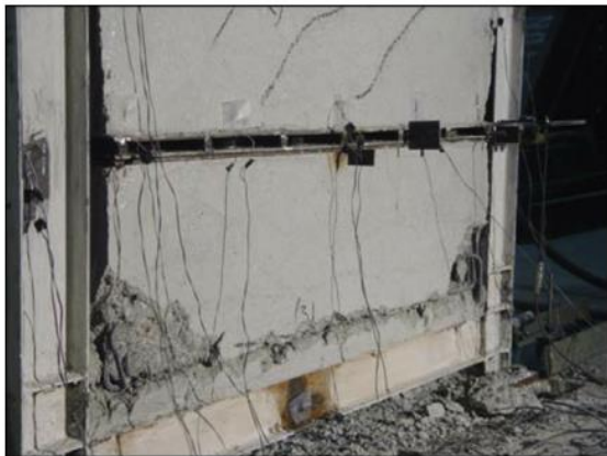
(a) Corner crushing and shear failure of infill.
