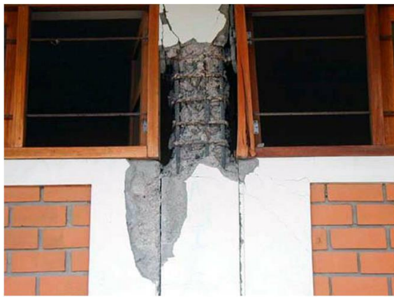
Fig. 2 Short column effect due to partial tight fit infill walls in an R/C building (Arequipa, Peru, June 2001 Earthquake, EERI) [11]
