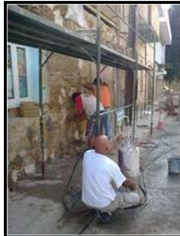
Fig. (20): An overflow of grout from holes at a higher level.
