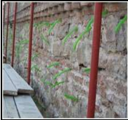
Fig. (18): Installation of a rubber tubes in the wall for the installment of the
