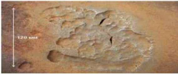
Fig.1 Corrosion damage on a pipe's wall [8]
