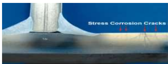
Fig. 9 Stress Corrosion Cracks on a pipe [35]
