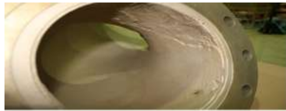
Fig. 7 Riser bend suffering from erosion-corrosion [33]
