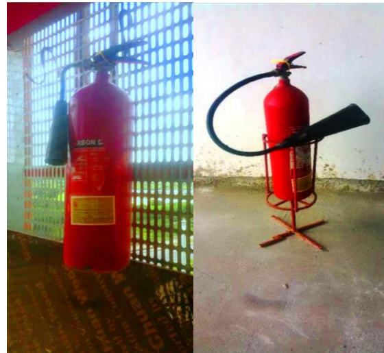
Plate #4.02; Fire extinguisher provided in a temporary lift and one of the floor of the constructed building, Source: Author, (2018).
